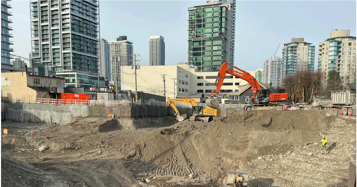
Jan 22, 2025 South West corner. Newly shot shotcrete panels (dark grey) at first row.
