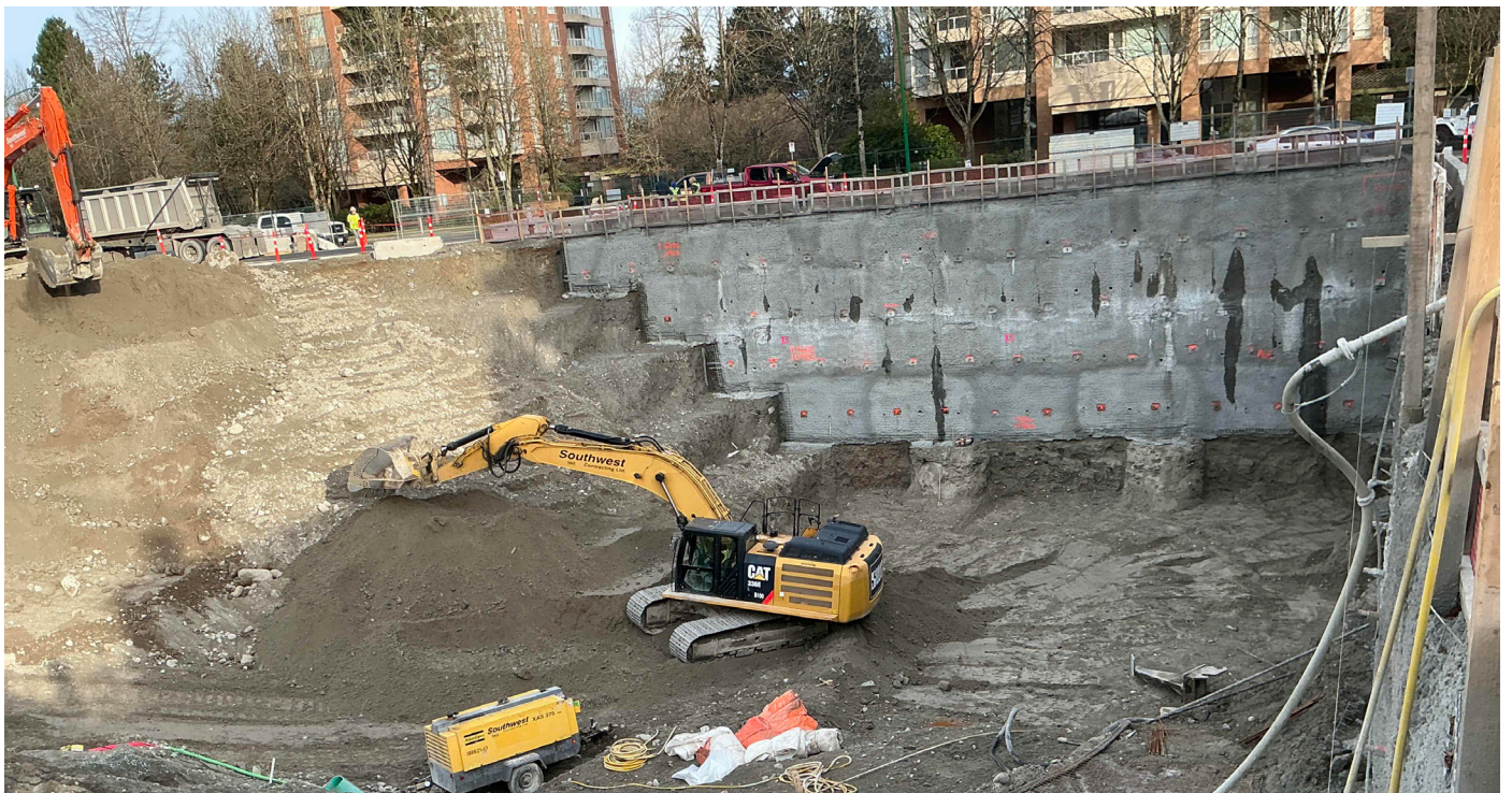
Jan 22, 2025 North East Corner. Four complete rows of shoring panels in place, working on 5th row. Excavated to approximately 30' below grade.
