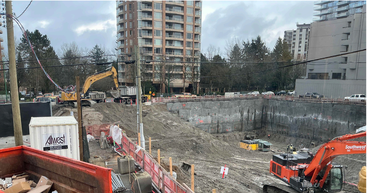
Jan 16, 2025 North East corner. Four complete rows of shoring panels in place, working on 5th row. Excavated to approximately 30' below grade.
