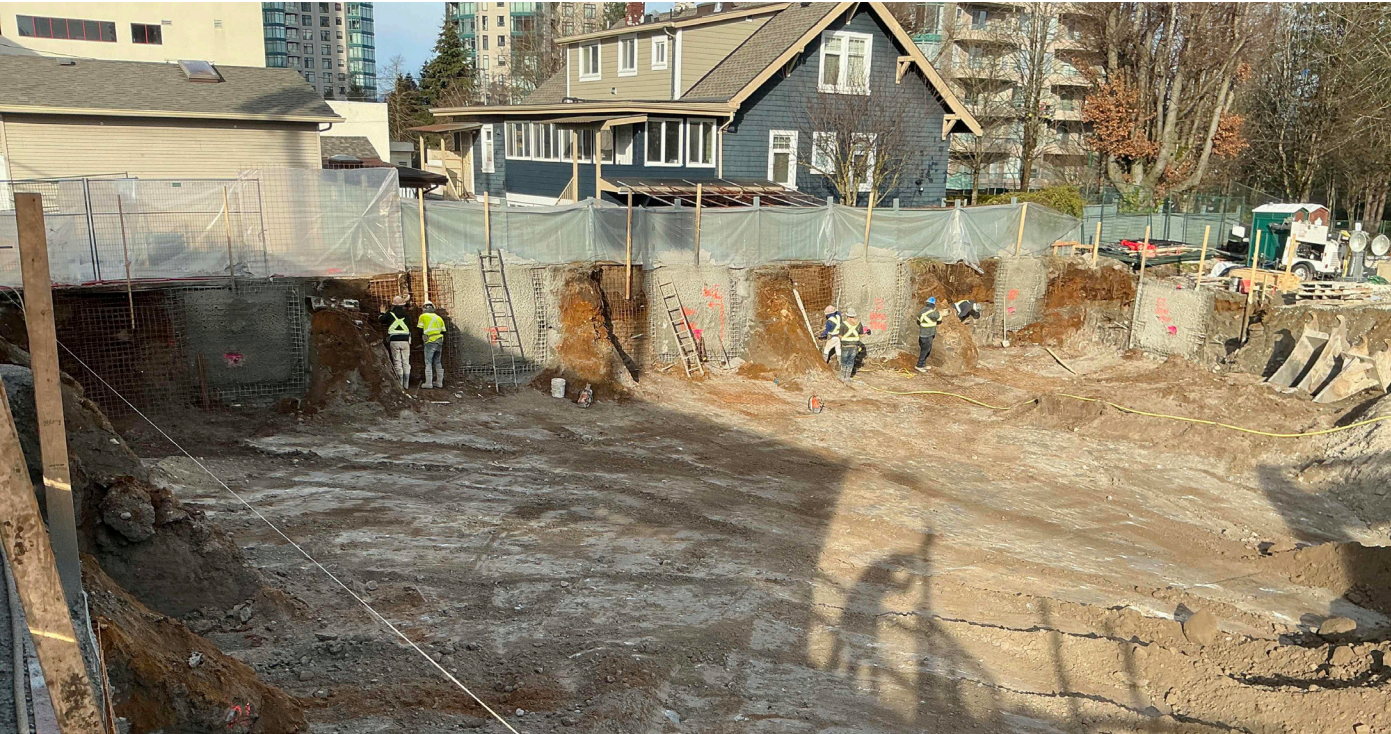
Jan 20, 2025 First set of shoring panels in place at West elevation. Preparing next set of panels for shotcrete.
